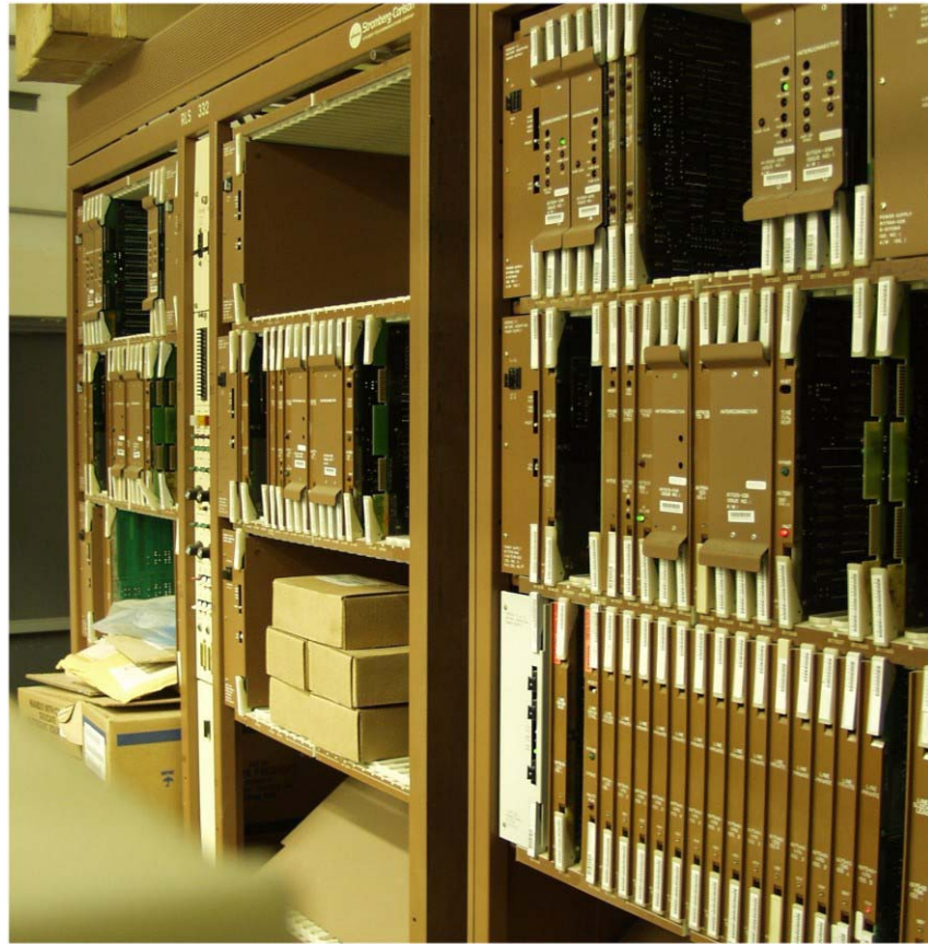
Figure 14-4: Equipment Rack with SLICs Inside an End Office
